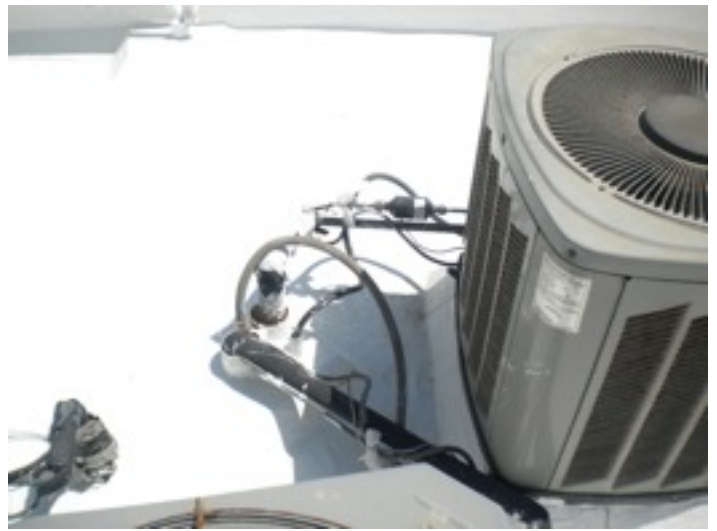
units missing insulation
