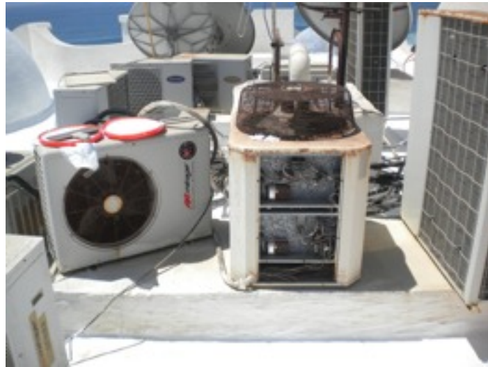
Building A/C unit
